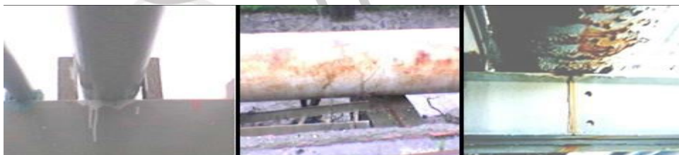
Fig 1.1 Pipe support locations, without sacrificial pads, in a refinery
